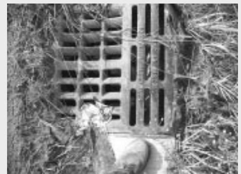
PHOTO by St. Joseph County SWCD: Typical plugging of filter fabric in inlet that is hard to clean
