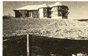
Silt fence can be an effective sediment control practice on individual lots during the house construction phase. They keep sediment from getting into the streets and street inlets, and from damaging neighboring lots.
