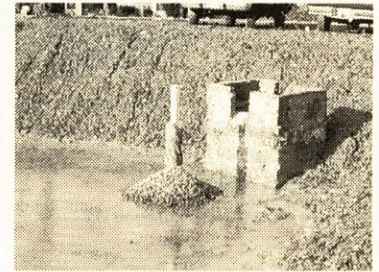
A slow release device installed in a stormwater detention basin detains water from the drainage area for up to three days.
